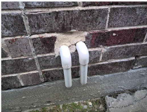
TPR Valve Drain Line
