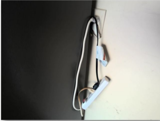
46. Extension cord used as permanent wiring was visible at the garage.
