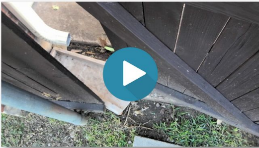
40. The fence door is obstructed by the downspout splash guard, interfering with its operation. This issue needs to be resolved.
