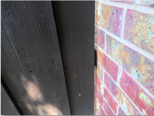
39. The wood fence is in contact with the exterior wall of the structure.
