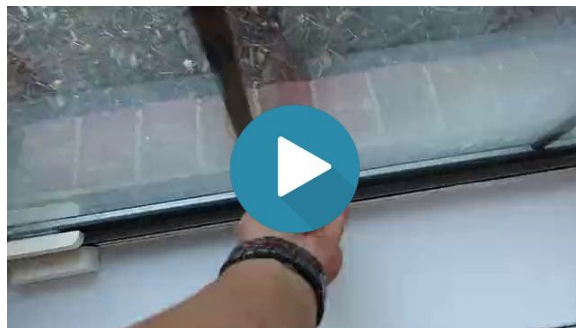
Windows are old, most window were difficult to operate and needed maintenance. Should consult with a qualified contractor to discuss options and costs for repair or replacement.
