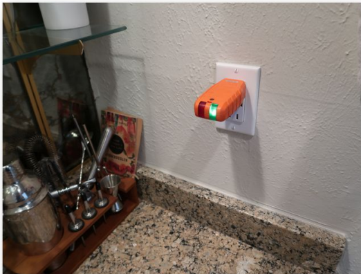
47. Electrical receptacles in the wet bar was installed upside down, with the ground holes above the neutral and hot slots.
