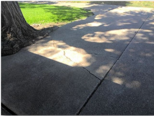
37. The driveway at the back of the house shows significant cracking due to tree roots.
