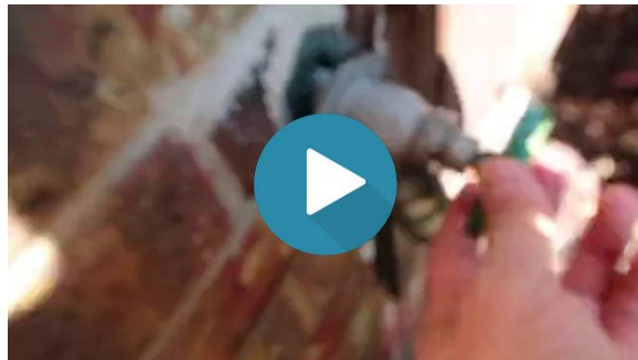
One of the exterior hose bibs is severely loose. It should be secured to prevent damage to the pipe.
