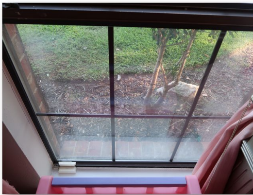
Front room windows are missing screen observed. An evaluation and work as necessary should be performed by a qualified contractor.
